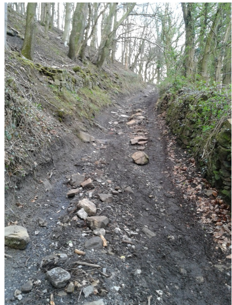
Surface and subsoil washed away, corner with limited visibility on Jacob's Ladder
